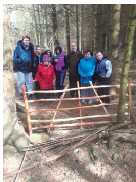
The completed gate is installed by the Thursday Bodgers out on the reserve
